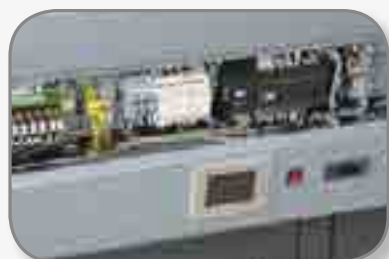
PLC ed elettronica: Made in Italy
